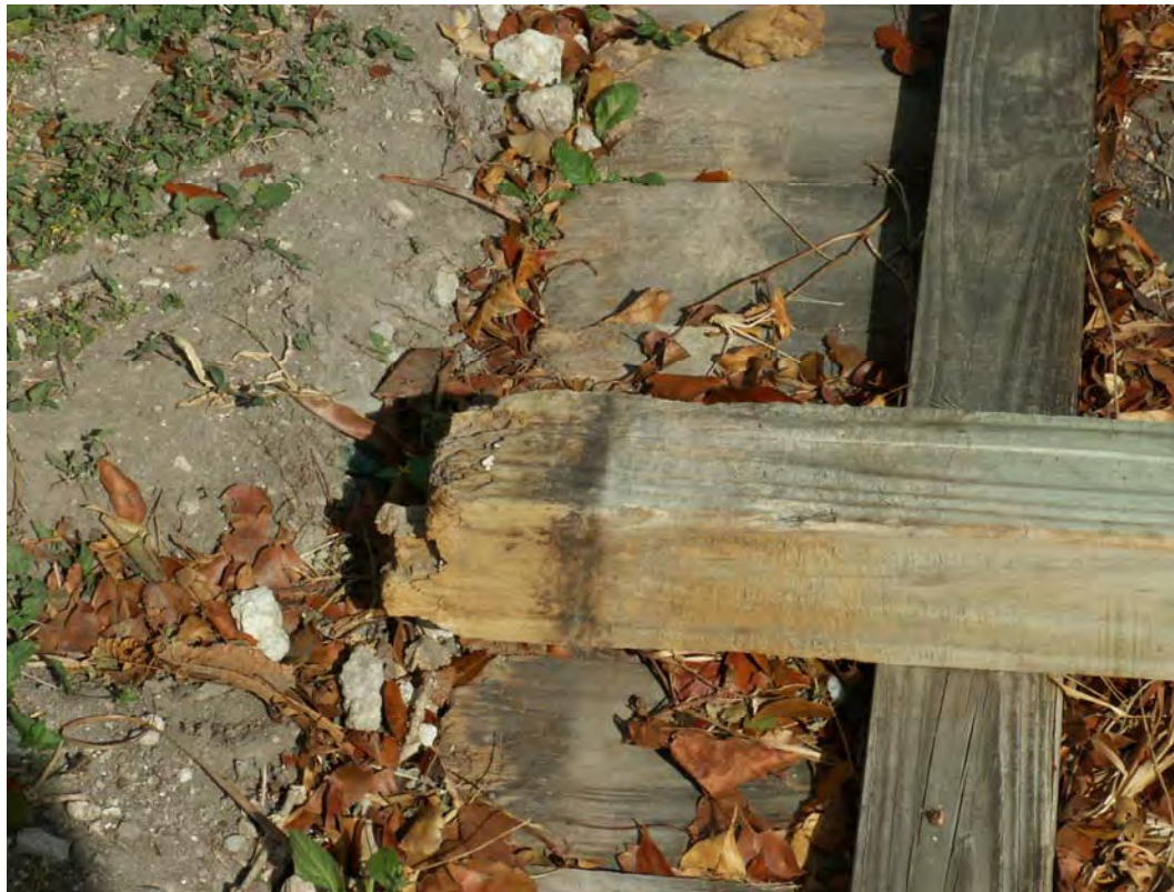
View of wood fence damage caused by obsolescence.
