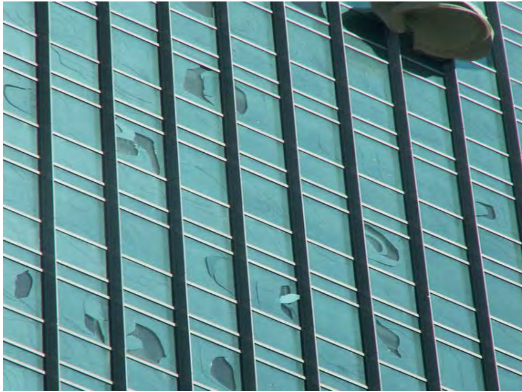
View of glazing damage in the Brickell area.
