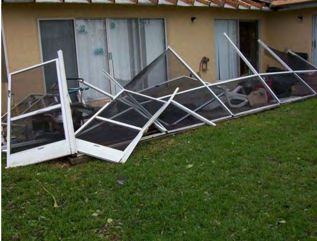
View of screen enclosure damage caused when screen panels did not break away.
