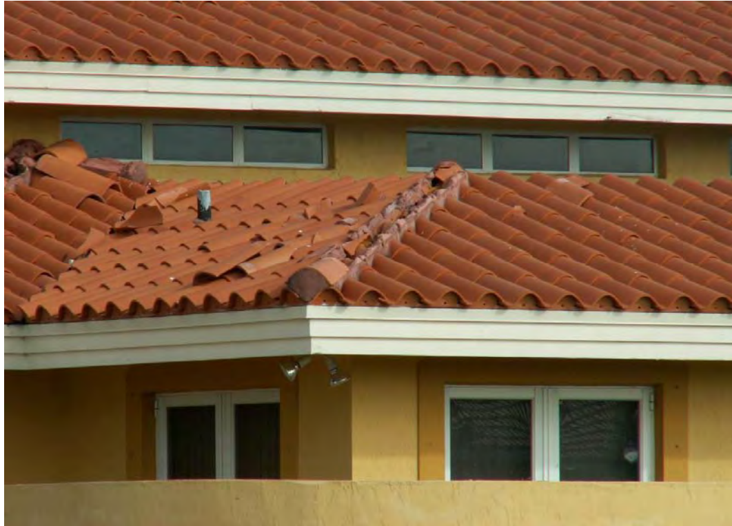
Typical view of hip cap wind loss on a clay tile system.
