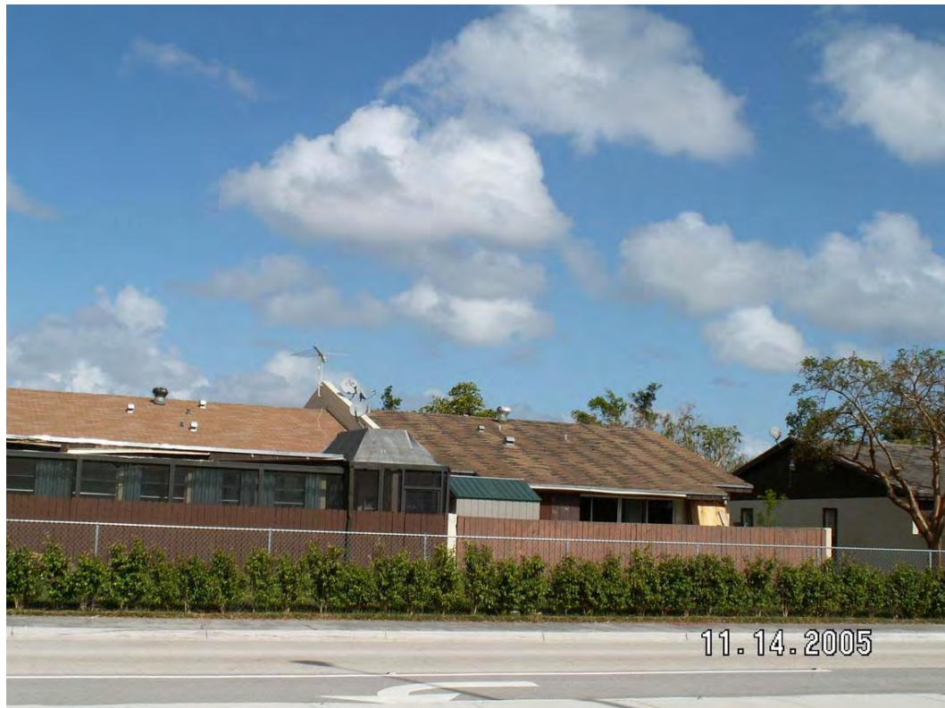
Side by side view, undamaged new shingle on the left. Damaged older shingle roof on the right.
