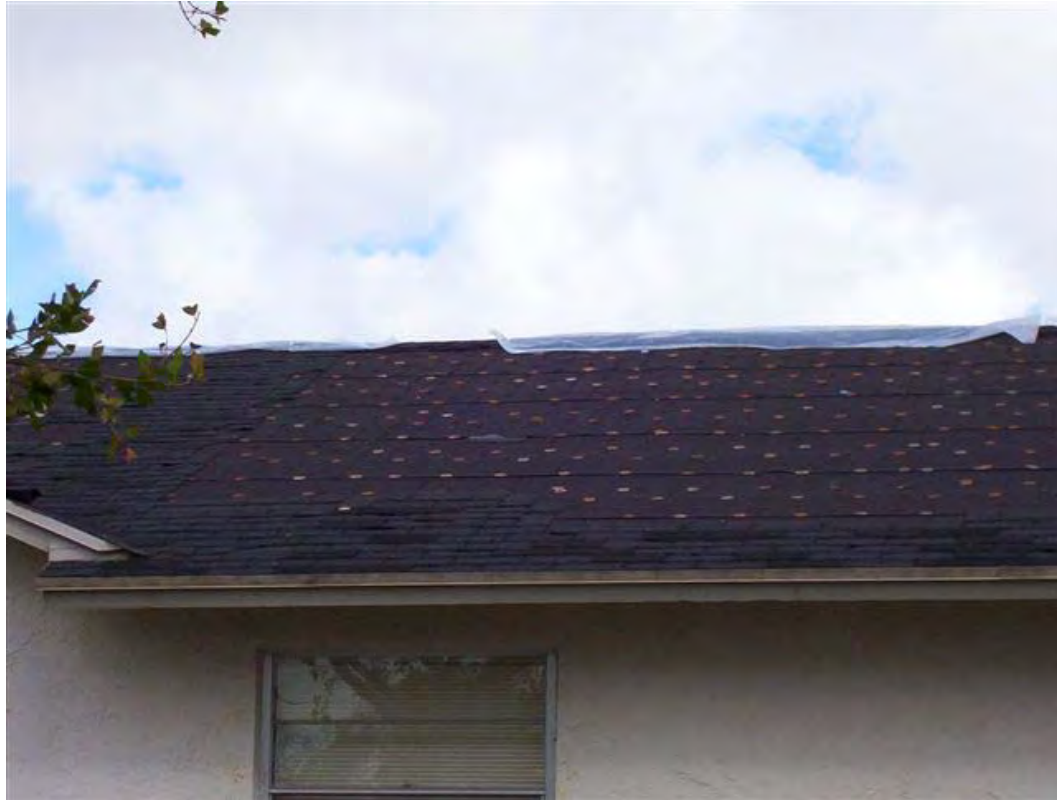
View of roof with shingle loss, with underlayment still in place.
