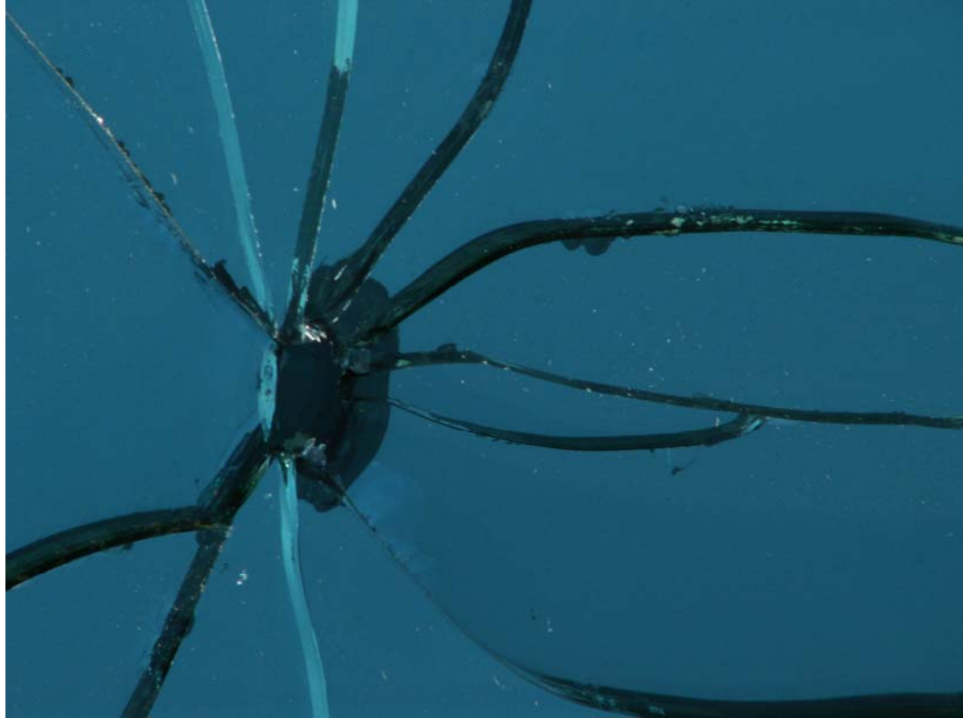
View of large missile debris impact above the 30 th floor.
