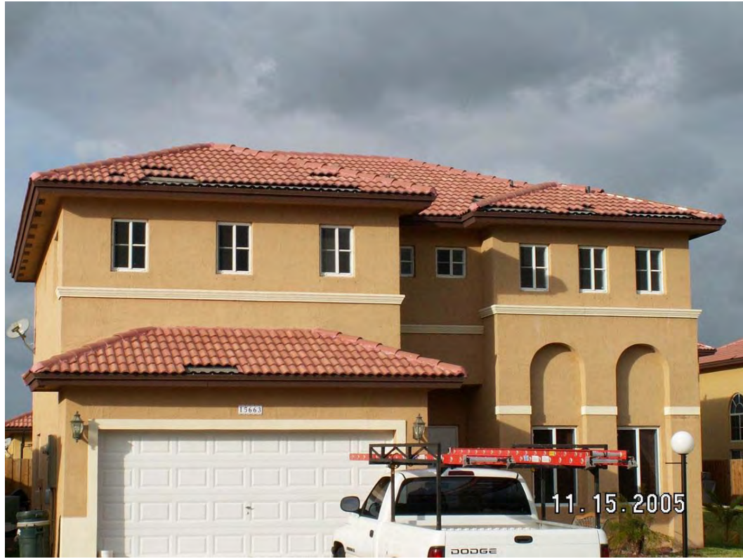
Typical view of first tile course wind loss.
