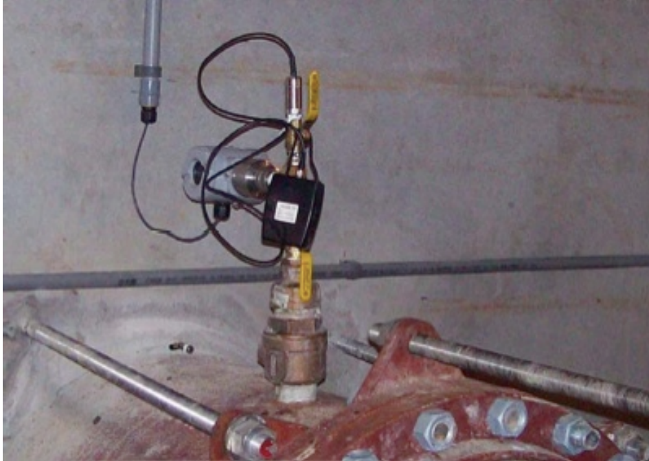
Figure 6-1 Example Pressure Logger Installation
